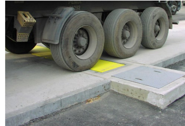
Proper construction of the weighing zone - road with cement concrete cover above the level of the surrounding terrain
