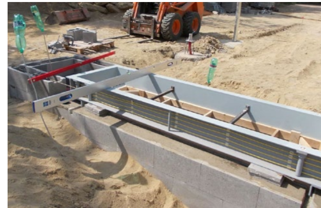
Monolithic base of scales using „lost formwork. The base frame of the scales is leveled on the base tray, to the left of the frame (towards the weighing room) the base for the inspection shaft can be seen.
